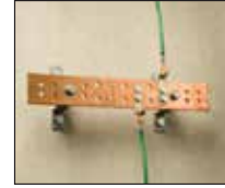
Telecommunications Ground Bar (TGB) and CADWELD Lugs
